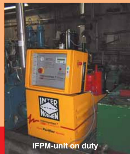
Off-line filtration on duty
